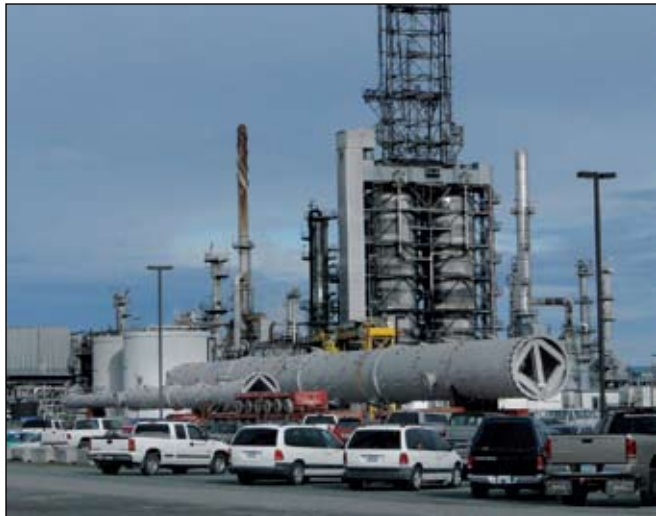
Columns at refinery ready for "dress out."
